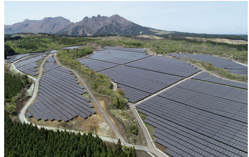
JRE Aso Takamori Solar Power Plant Project
