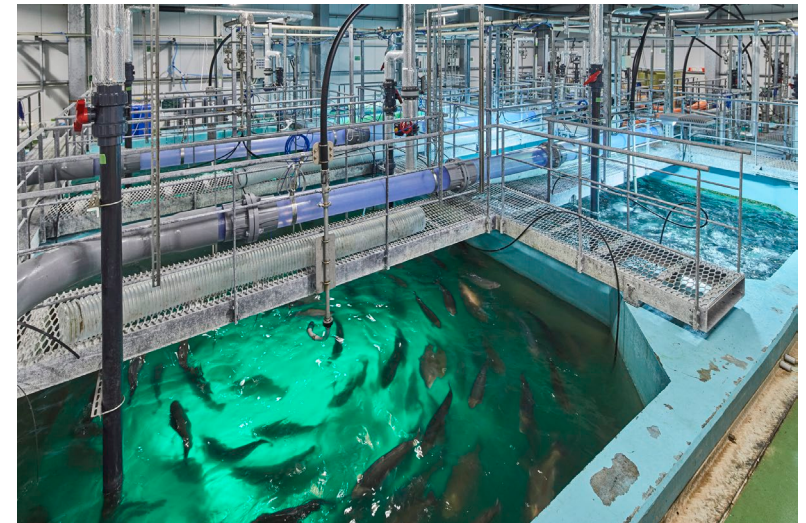
▲ Closed recirculating land-based aquaculture system in operation
