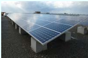
Project in Ishikawa Prefecture (Solar panels)
