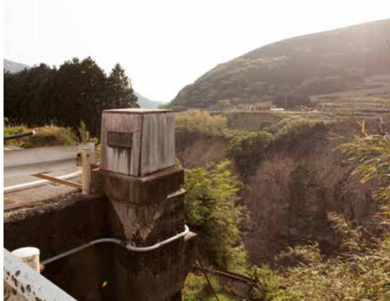
Tateno district cut off by collapse of Aso Ohashi Bridge due to landslides
